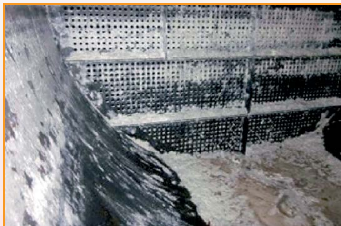
Prior to NoWax application. Production facilities plugged with wax.
